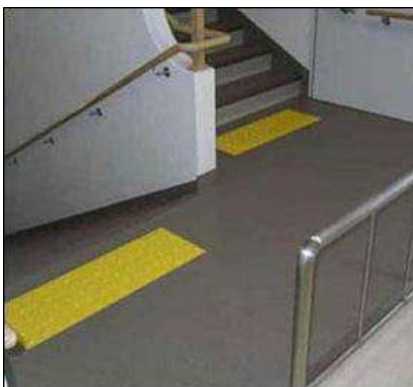
Figure 7-9: Warning blocks at landings
